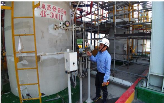
04.2018 Process safety assessment on liquid ammonia tank at a cogeneration power plant, project manager Chyuan Lee.
